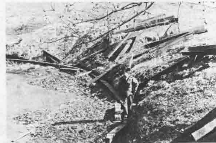
Workers are shoring up the banks of Bugg Lake with railroad ties in an effort to stop erosion.
